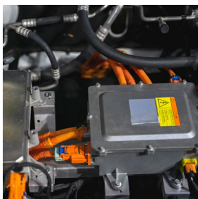
Battery Management Systems
